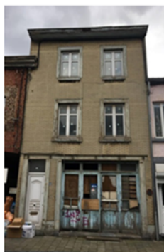
B. Need of heavy renovation
