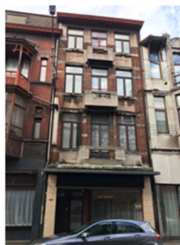
C. Need of maintenance
